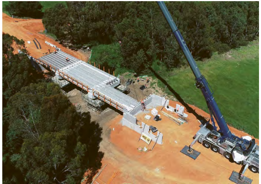
Above : Aerial view of the progress work on the Franklin Bridge, looking towards Buninyong on 10 November 2020 showing the heavy duty crane lifting and placing the massive concrete beams that form the bridge.
