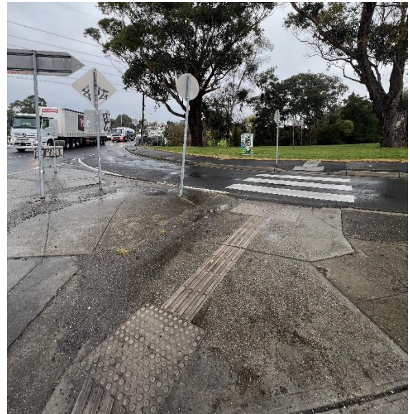
Nicholson Street western slip lane (Bell Street left into Nicholson Street movement)
