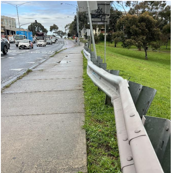
Damaged collision barrier on north-west aspect
